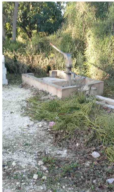
Fig. 4 — Abandoned and deteriorated pump
