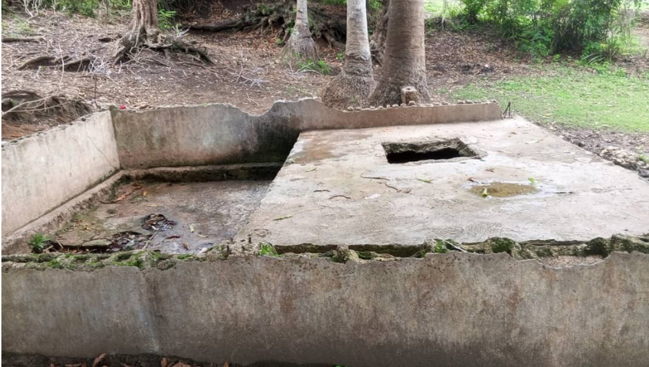
Fig. 1 — Destroyed water intake reservoir, former main supply point (pre-2010)
